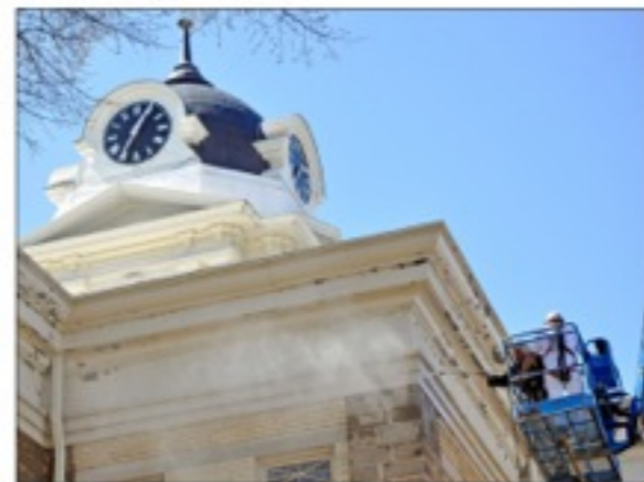
Prepping for painting CARROLLVILLE - Contractors blast off old paint from the Franklin County Courthouse Monday. Work began this week to repaint the courthouse. All of the painted surface on the courthouse, save the dome at the top, will be repainted. The painted areas of the building are actually metal, County Manager Sid Morse said. The county is using special purpose local option sales tax funds for the work. Davis' Painting of Franklin County was awarded the bid for the work, which should take a few weeks.
