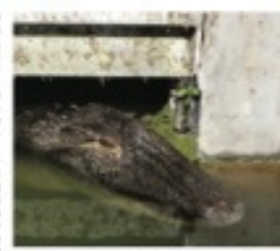
This 7-foot-3-inch alligator found its way into the contact chamber of the city's waste water treatment system last week.
