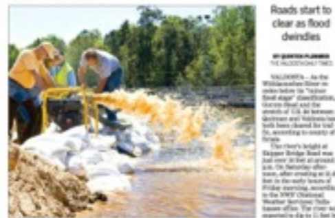
In this 2009 photo, city workers and volunteers set up a portable water pump on top of the 10th station of the wastewater treatment facility. The pump was used to pump water out of the 10th station and into the river. The pump was used to pump water out of the 10th station and into the river.
