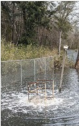
A section of the discharge pipe at the plant is currently underwater.
